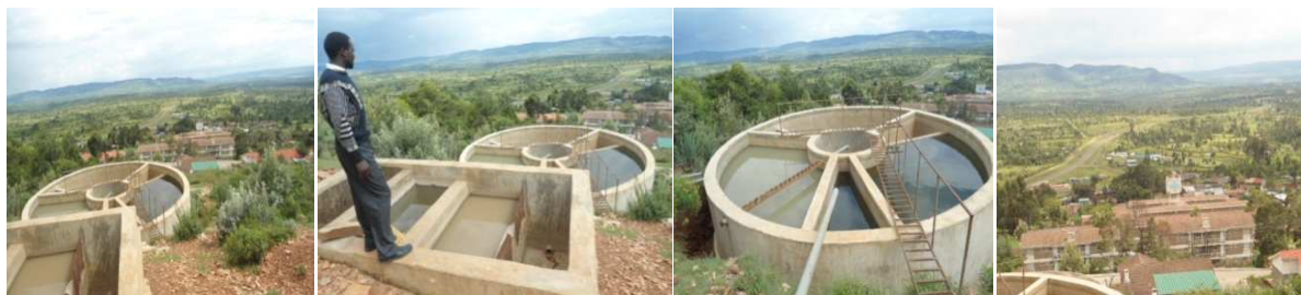
Photo 2.4: Longisa water treatment works
